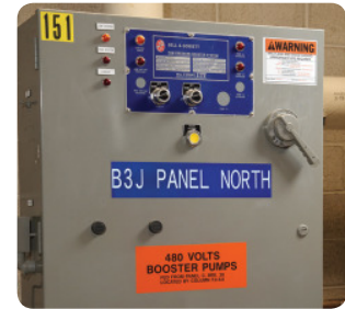
Control Panel & Electrical Panel Labels
