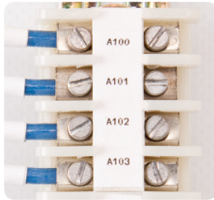
Terminal Block Markers
